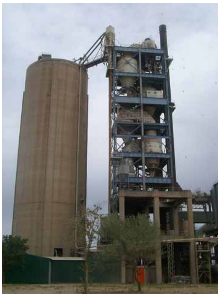
Figure 2-6: Photograph of the 5-stage preheater of Kiln 1 at Dwaalboom. The raw meal silo is located to the left of the preheater.
